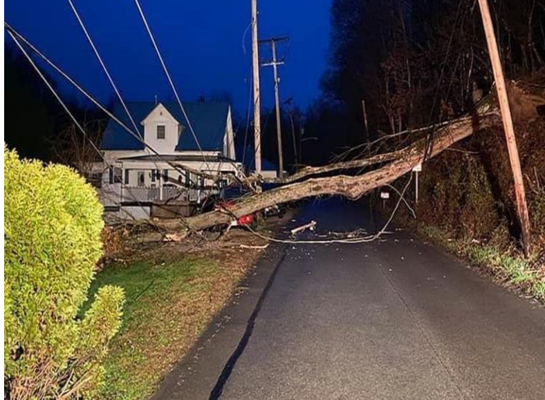
Figure 25: Damage From High Thunderstorm Winds
